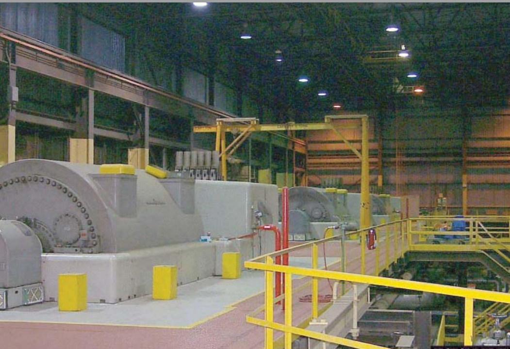
Level 2 generators with VESDA Sampling Pipe in protected area, and detection unit mounted in a control room for ease of maintenance access.
